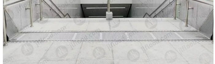
Recessed channel & drain grate, embedded install
