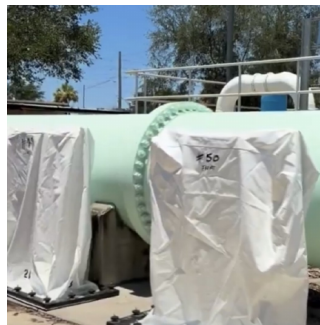
VALVE ASSEMBLIES, INDIVIDUALLY COVERED
