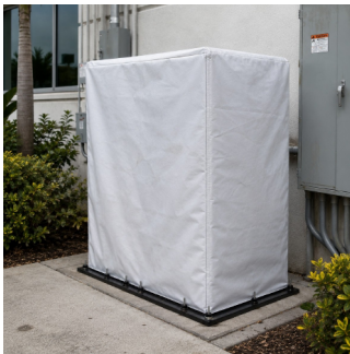
PAD-MOUNTED ELECTRICAL EQUIPMENT
